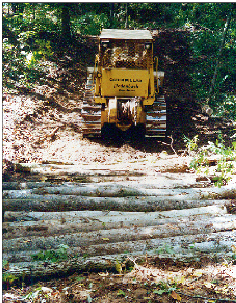
Figure 23B. Pole crossing.
